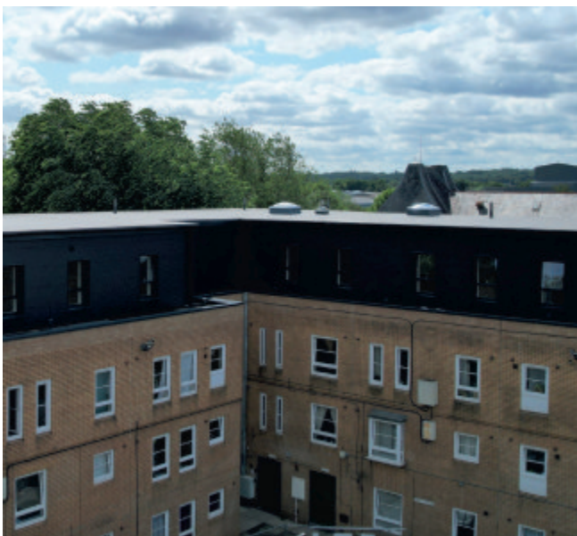
Ten new apartments have been added to Dover Court (pictured), as well as Woodstock
